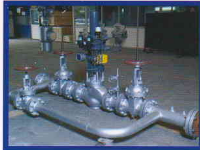
Pressure reducing cum desuperheating station
